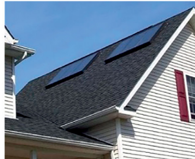
Roof-mounted solar heating
